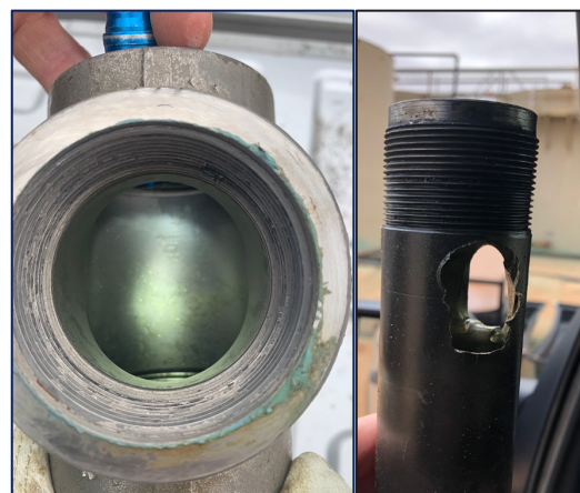
Left: Blaze treated Tee after December 2020 inspection. Right: Damaged cage during December 2020 offset frac.
